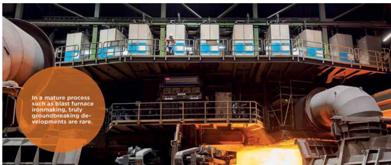
Fig. 1: Image showing a blast furnace with SIP installed. The proprietary SIP boxes can be seen in the upper part of the picture (silver/blue)
