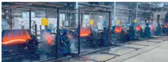
Fig.4: Roughing Mill Train with F-MTC
